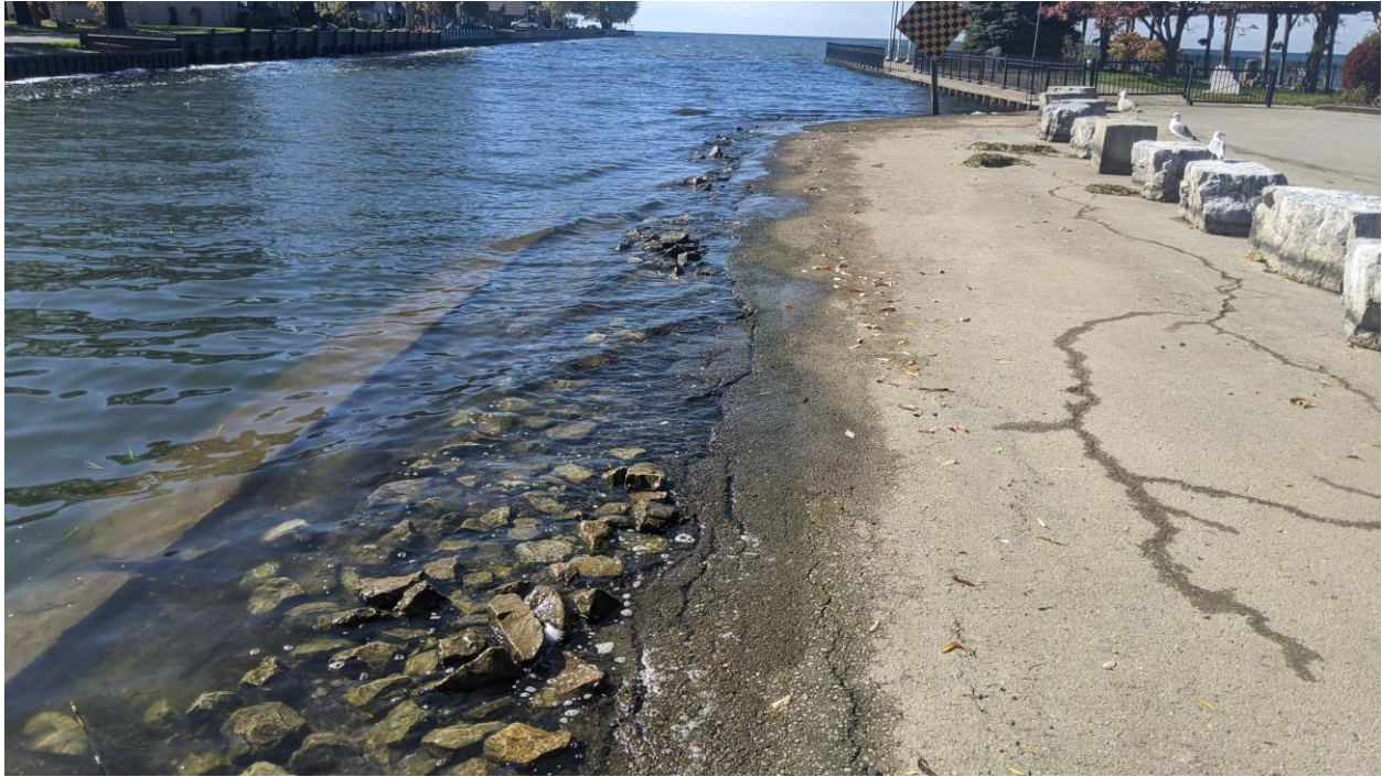
Figure 2. Mitchell’s Bay Retaining Wall – Submerged Top of Retaining Wall and Deteriorated Edge of Asphalt
