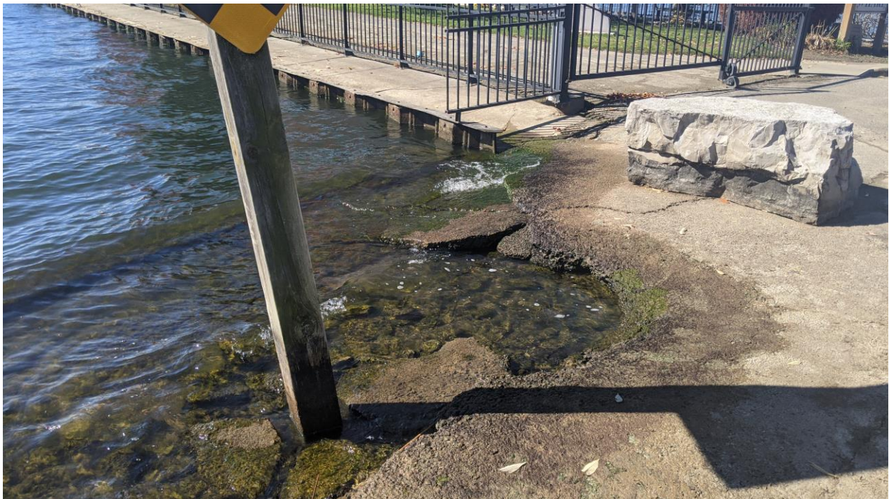
Figure 3. Mitchell’s Bay Pier – Settlement of Existing Concrete Retaining Wall Adjacent to Pier Sheet Pile Wall. Deteriorated Edge of Asphalt and Loss of Material
