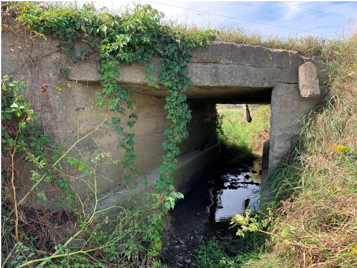
Figure 1. Base Road over Morgan Drain – East Culvert End with Spalled/Hanging Concrete and Overall Deterioration
