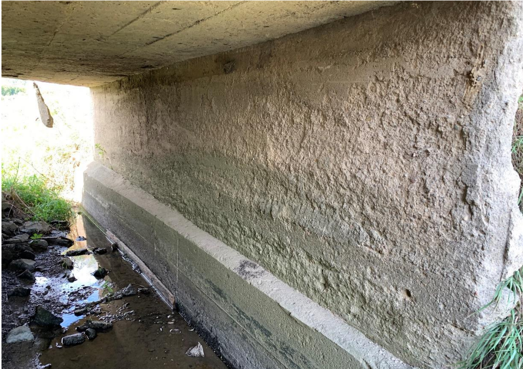
Figure 2. Base Road over Morgan Drain – Interior Culvert Surfaces with Severe Scaling, Delamination, Spalling, and Exposed Footing
