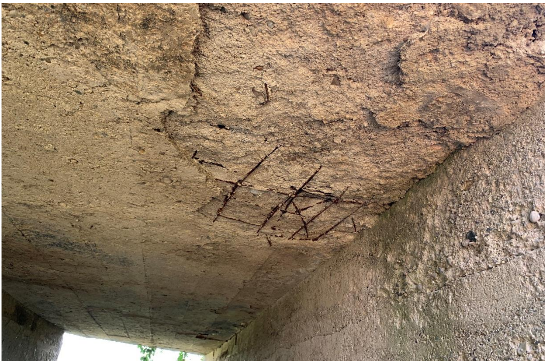
Figure 3. Base Road over Morgan Drain – Soffit Deterioration with Exposed Corroded Reinforcing Steel
